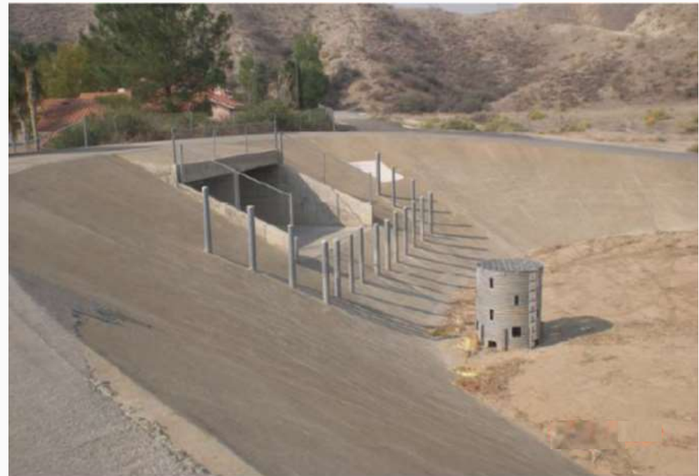
Debris Retaining Inlet
